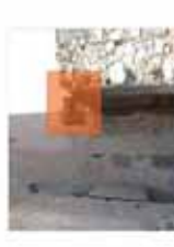
Identification of the base surface is a key step in the process. The orange marker indicates the location of the wall. The wall is curved and the marker is placed on the wall.
